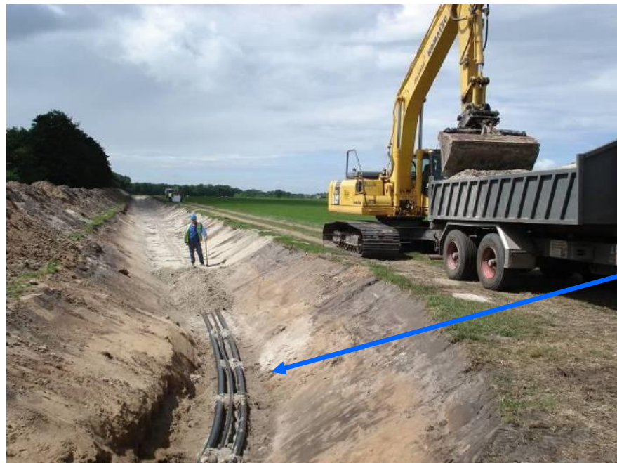
Installation of high capacity XLPE insulated DC cable system in rural area in Germany
