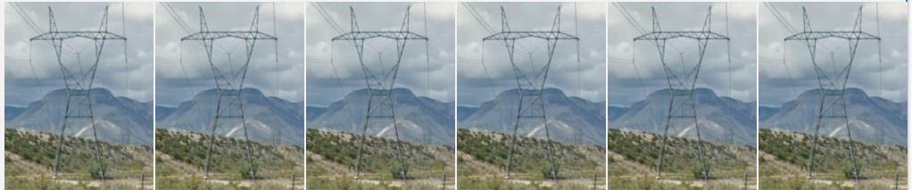
6 - 345 kV Single Circuits
