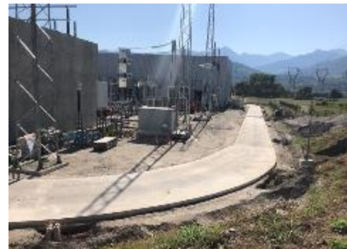
Converter station at Piosasco
