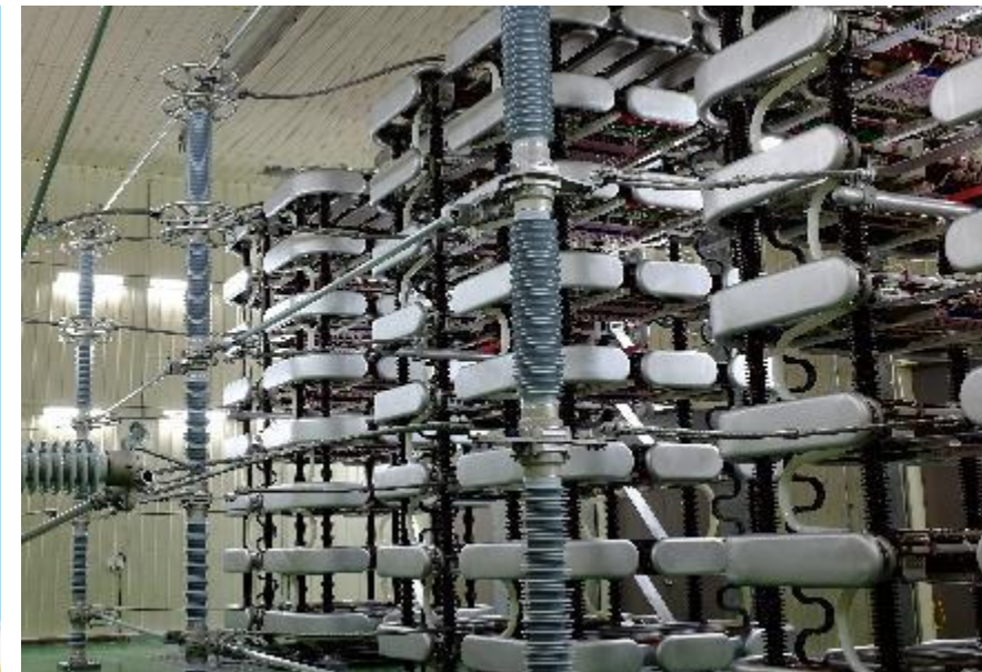
H450 Valve Installed in Converter Station
