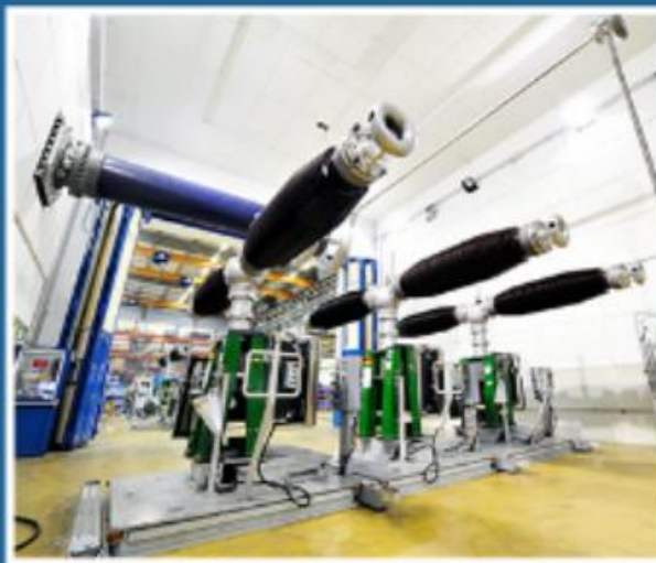
High voltage testing laboratory for internal routine testing according to international standards
