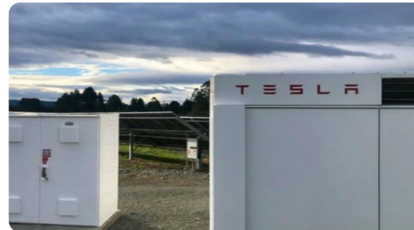
Redwood Microgrid—CA, USA
